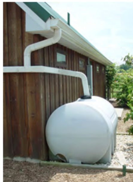
Cistern for harvesting stormwater that drains from the roof.
